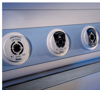
SmartLet monterat i vårdrumspanel
