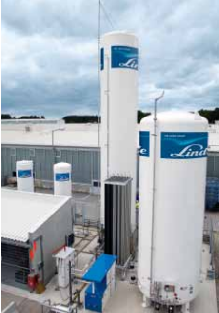
Figure 18: Storage tank and vaporiser for liquid nitrogen
