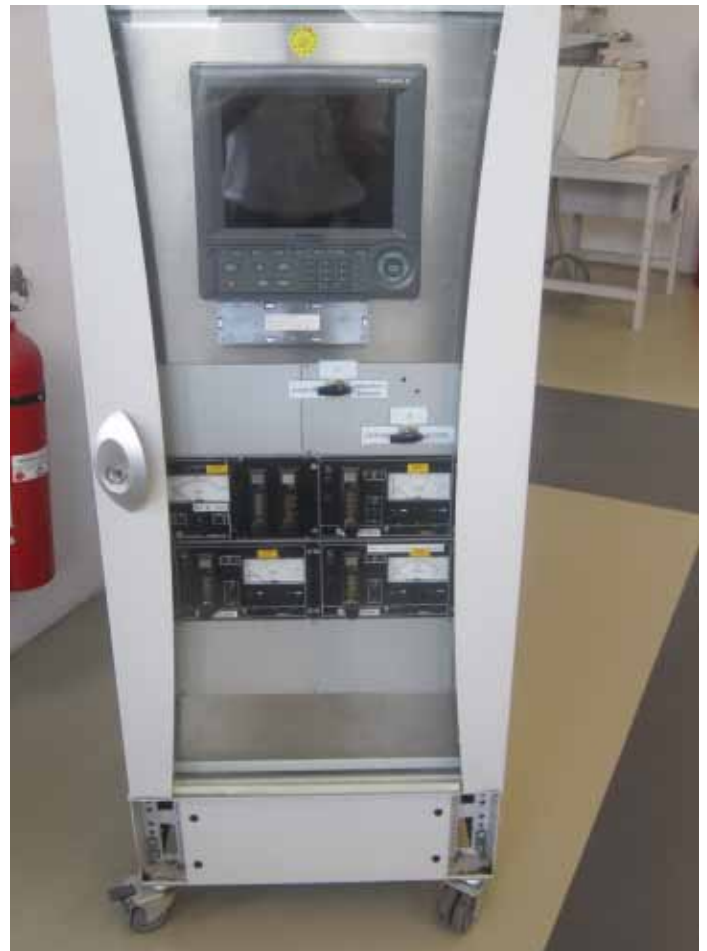
Figure 62: Analysis cart incorporating units for computerised data handling (upper part), sample gas handling with pump and valves, and gas analysers for hydrogen, methane, carbon monoxide and carbon dioxide (lower part)
