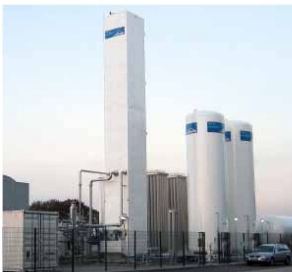
Figure 20: Cryogenic nitrogen production with CRYOSS®
