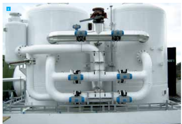
Figure 22: Nitrogen supply methods. a) Storage tank and vaporiser for liquid nitrogen, b) Cryogenic nitrogen production with CRYOSS, c) PSA (Pressure Swing Adsorption); ADSOSS.
