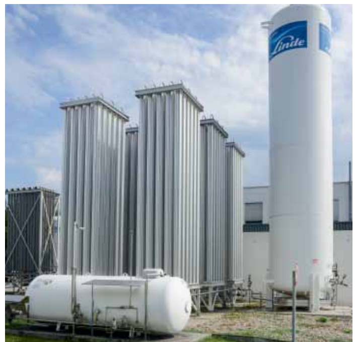
Figure 24: Methanol tank installation. The liquid nitrogen tank is seen in the background.
