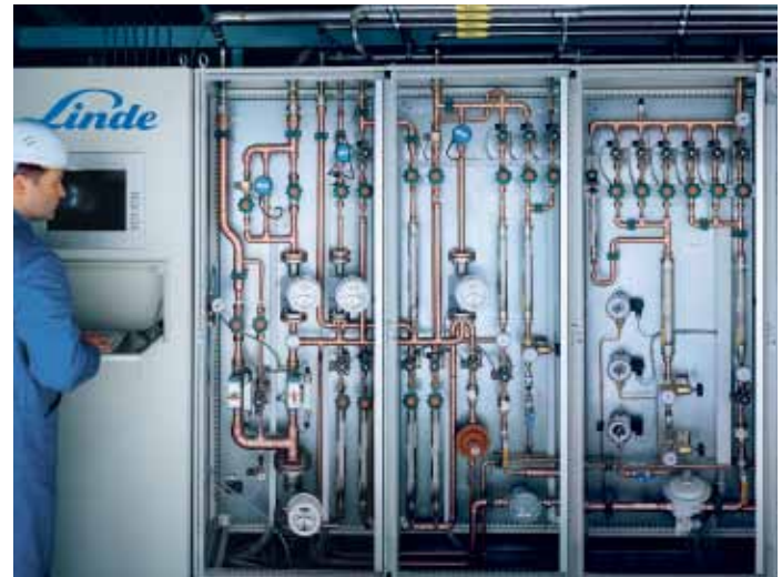
Figure 46: Example of a control cabinet for a nitrogen/endogas system
