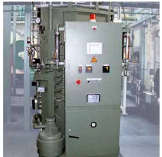
Installation of an external endogas generator (photo courtesy of Ipsen)
