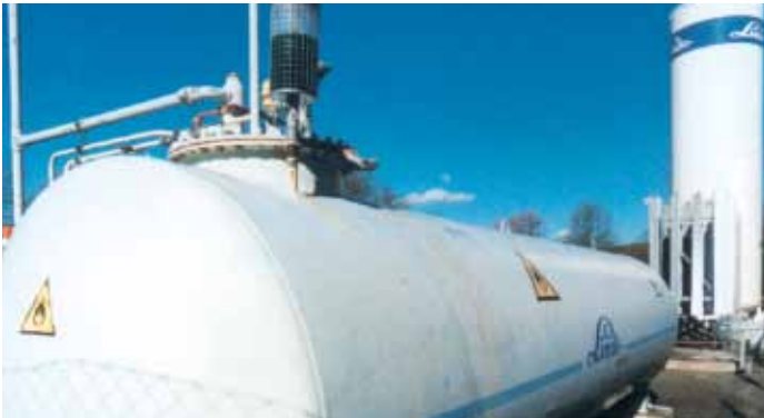
Figure 25: Methanol tank installation. The liquid nitrogen tank is seen in the background.
