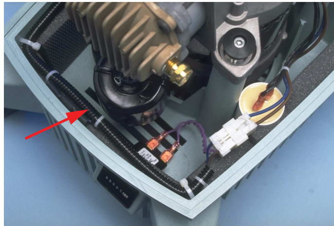
FIGURE AG: LOCATION OF THE MAIN POWER WIRING HARNESS
