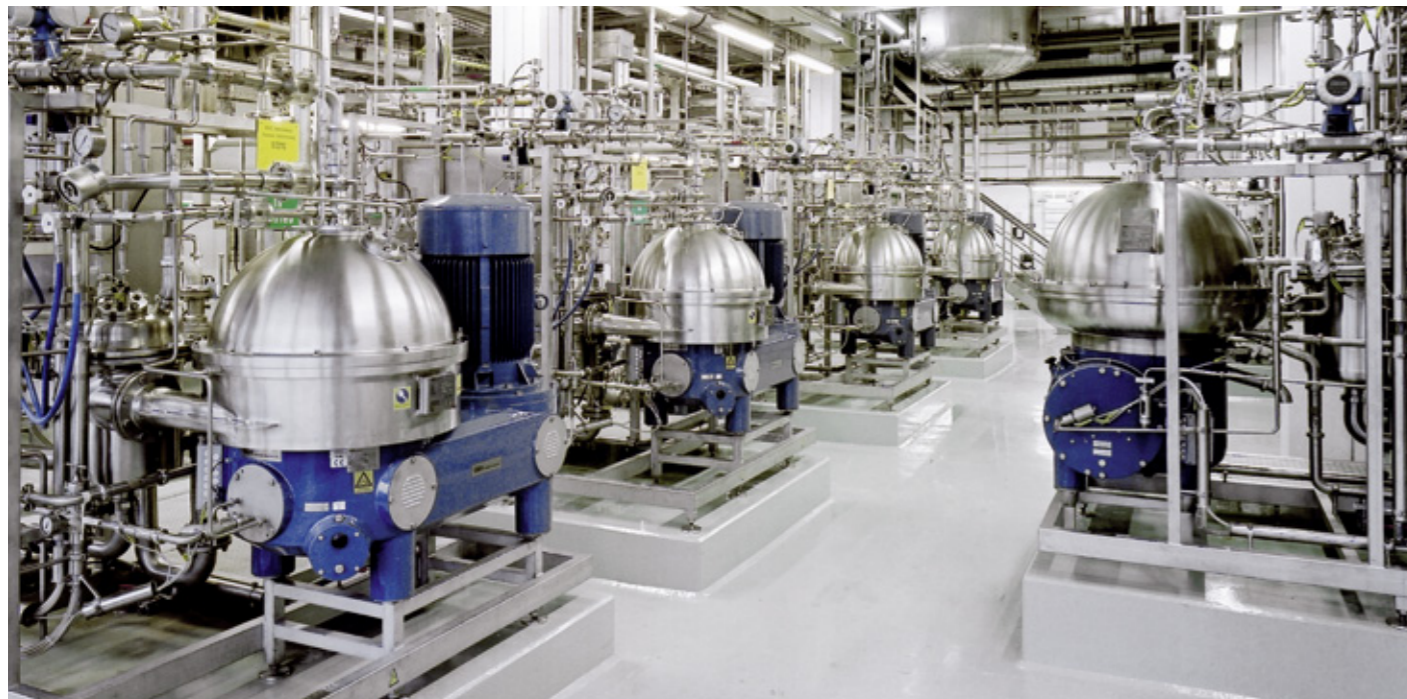
Interior of a large-scale biopharmaceutical plant, designed and constructed by Linde-KCA-Dresden.
