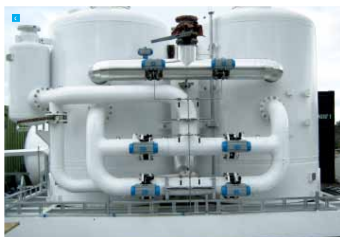
Figure 15: Nitrogen supply methods. a) Storage tank and vaporiser for liquid nitrogen, b) Cryogenic nitrogen production with CRYOSS ® , c) PSA (Pressure Swing Adsorption)
