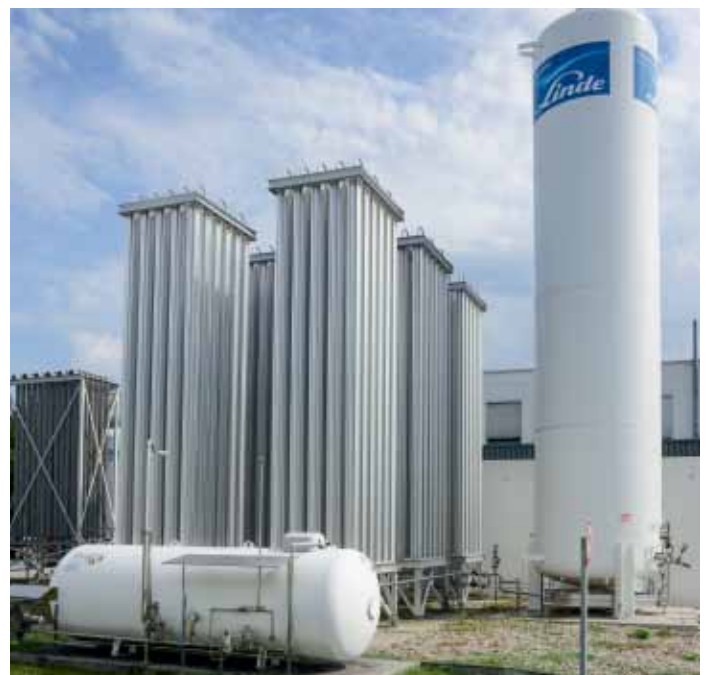
Figure 17: Methanol tank installation. The liquid nitrogen tank is seen in the background
