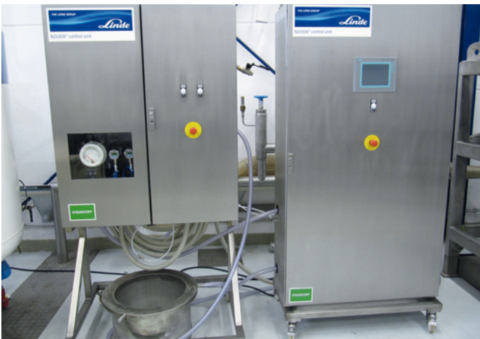
A measuring and metering station for the inerting of mixers or reactors
