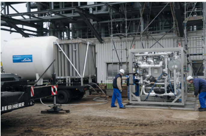
Installation of the mobile CRYCON® test unit at customer's site. Convincing test results led to an order of a customised cryocondensation unit.
