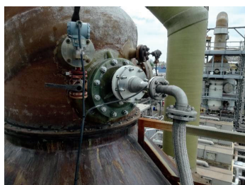
Figure 6. Ozone injection port
