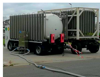
Figure 4. Oxygen storage, evaporation and pressure control equipment (Linde AG)
